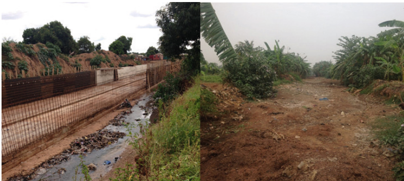
Figure 15.6 Reconstruction of a gutter in central northeast Tamale (left) and its end point 7 km outside the city centre (right). (Source: Imogen Bellwood-Howard)
