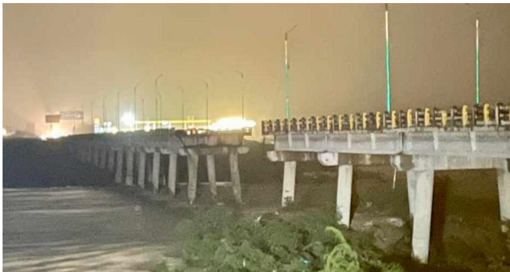
Hub river bridge destroyed cutting off Karachi road access to Balochistan
